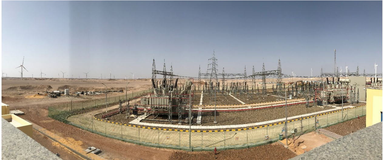
View on the 220 kV substation
