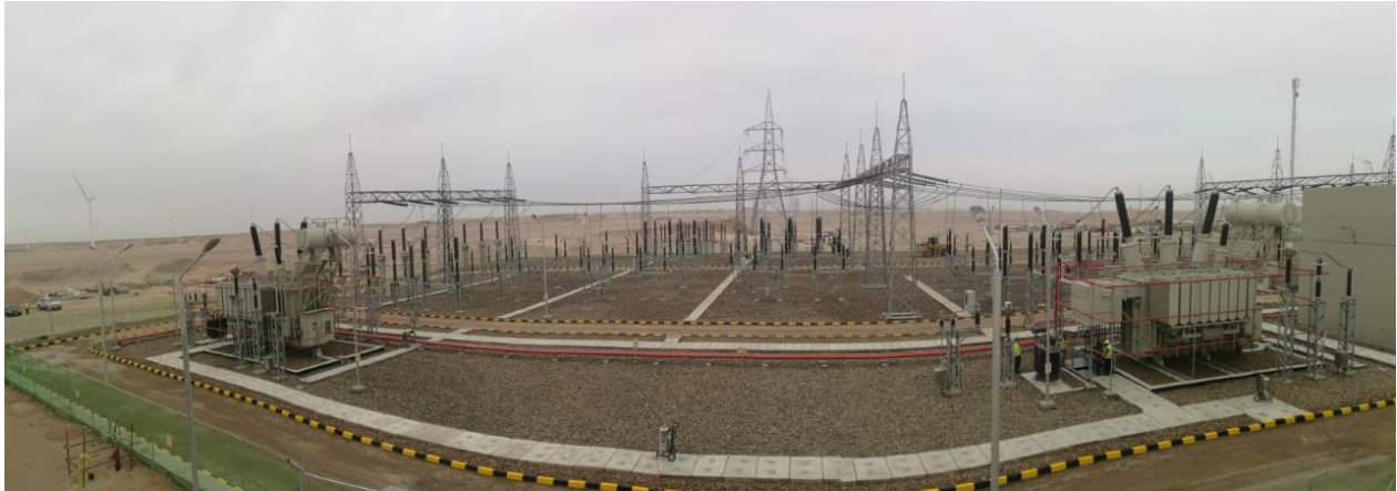
Substation was energized on April 15 th 2019
