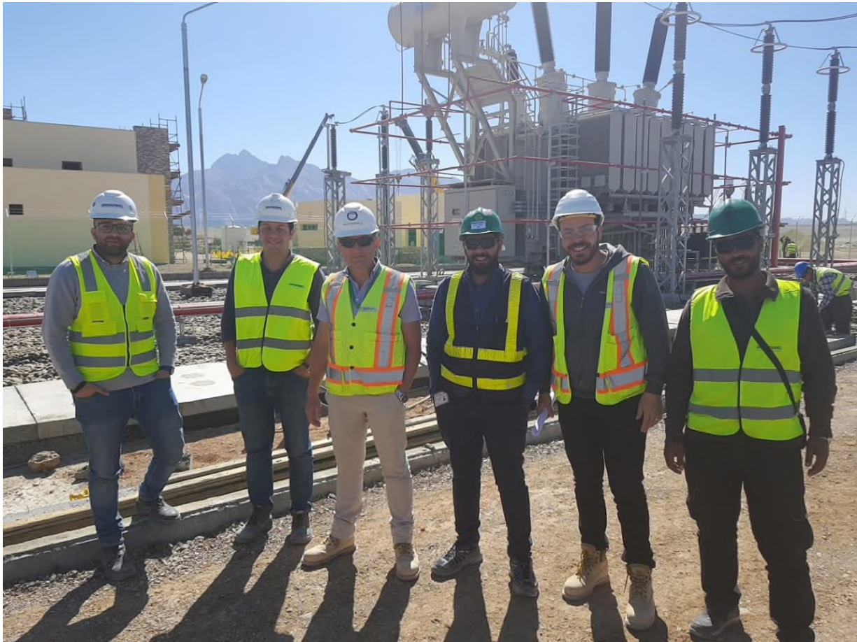
Project team members in front of 1 of the 3 main transformers, just before energization
