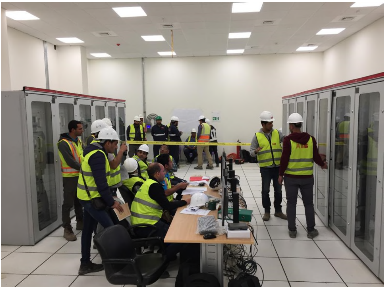
All the project team mobilized in the control room for the energization
