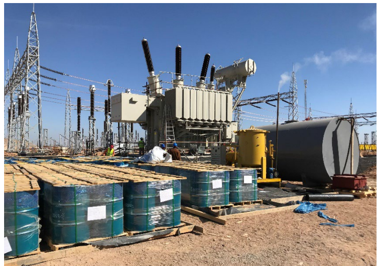
Oil filing of step-up transformer 1
